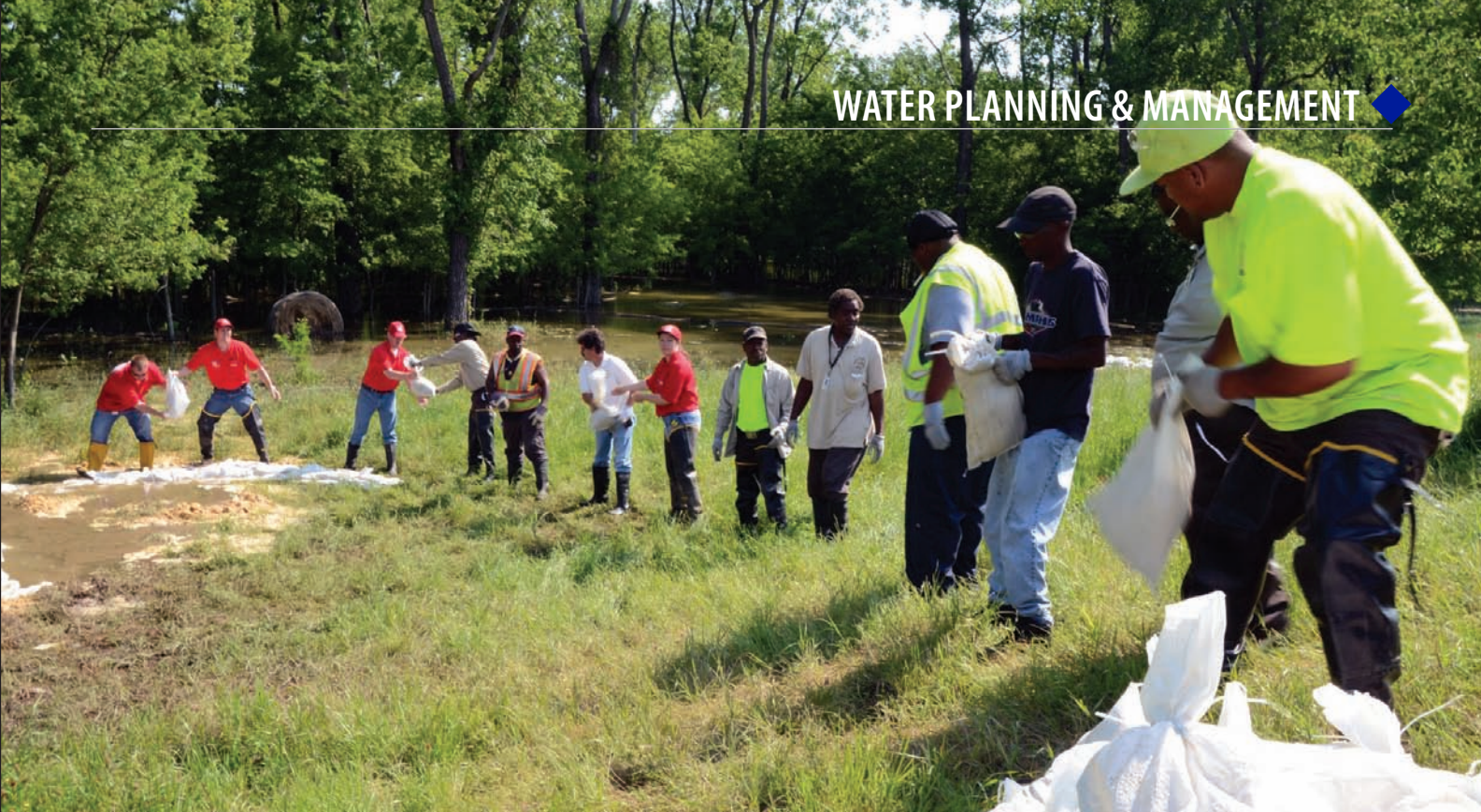
Members of the U.S. Army Corps of Engineers Memphis District and City of Memphis officials place sandbags on a sand boil in Memphis, Tenn., in May 2011.
